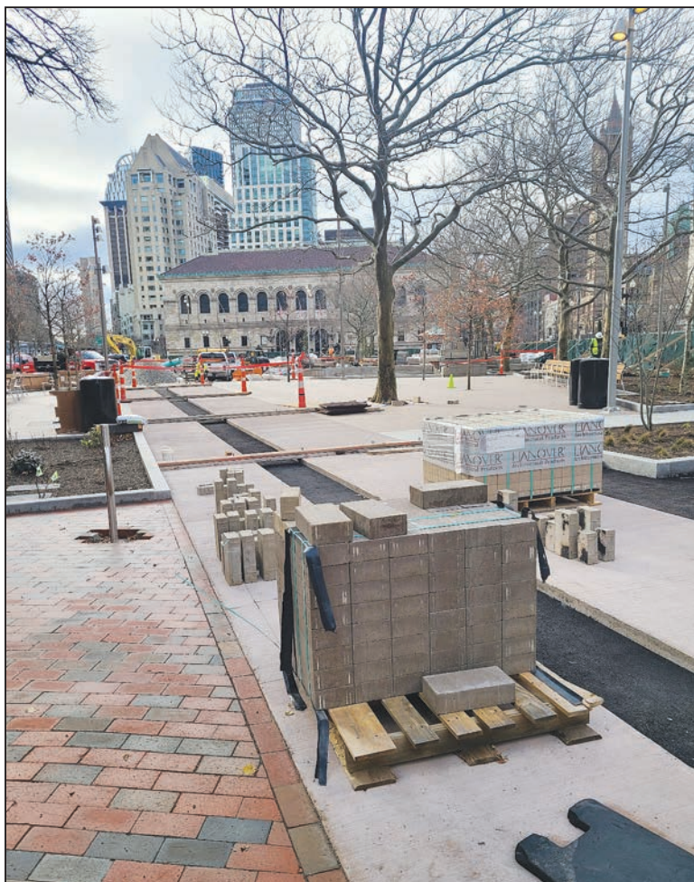
Looking southwest from the area we'll be opening shortly, north of Trinity Church, you can see the final pavers about to be installed on top of the asphalt stripe. The joint materials (with orange cones) are being protected from the rain. A new bike rack (on the left) needs to have bricks reinstalled around its base.
